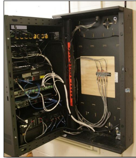
Fig 1: A properly wired equipment cabinet allows for easier service & operation.
